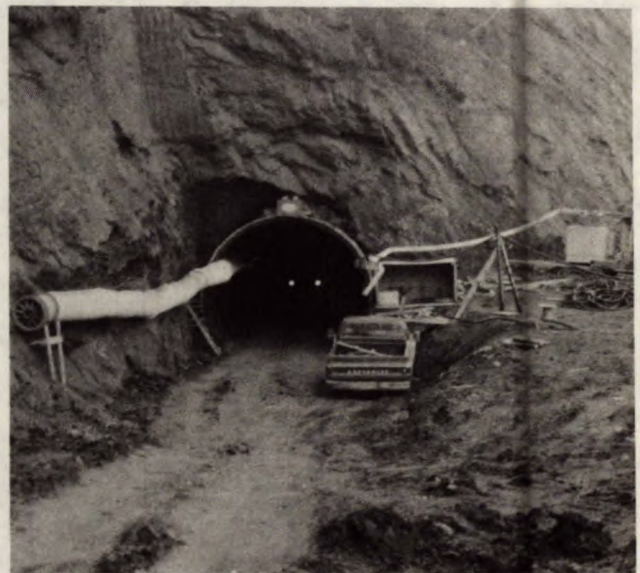
Figure 5 — The Saline Creek Diversion Tunnel — the first underground excavation in oil sands.
