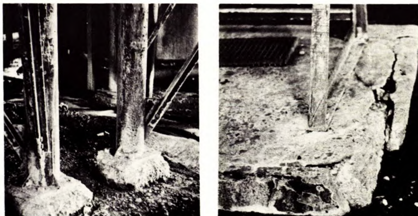
Fig. 2 - Deterioration of portland cement mortar in the concrete footings of a \text{Na}_2\text{SO}_4 plant, after 6 years. The aggregate rubble is sound, except for minor damage of schistose material. A protective concrete shielding (right) slowed the reaction greatly for a time.
