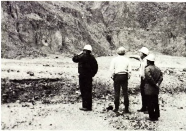
Fig. 5 - Some 4 ft (1.2 m) of heave beyond the toe of a 300-ft (91-m) wall
