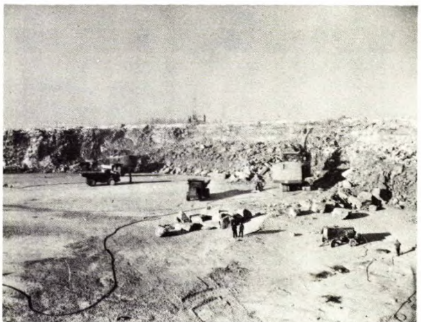
Fig. 6 - An upheaval of 8 ft (2.4 m) and cracking of the floor in an open pit during stripping indicated the presence of high horizontal stresses in the formation
