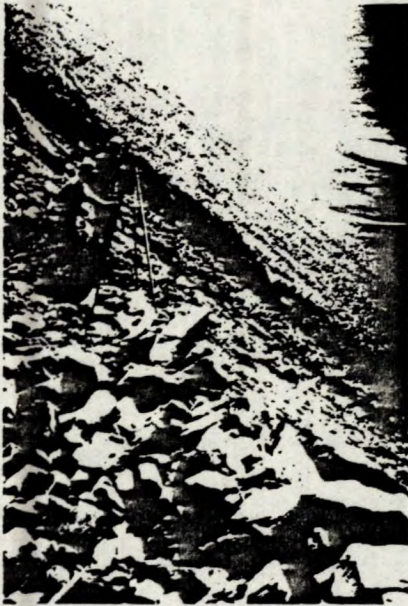
Fig 21 - Photograph of a pulley support unit installed at the crest of a waste dump.
