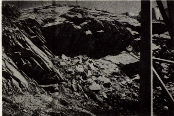
Fig 35 - Typical 3-d-wedge instability. Movement occurred along the two joint sets oblique to the face. The overhanging face is parallel to the bedding.
