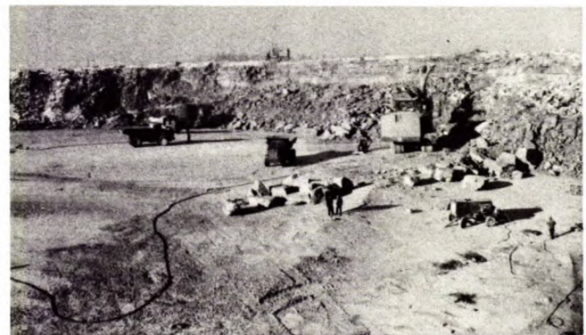
Fig. 37 - An upheaval of 8 ft (2.4 m) and cracking of the floor in an open pit during stripping indicated the presence of high horizontal stresses in the formation.
