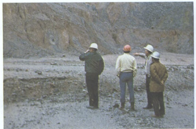
Fig. 35 - Some 4 ft (1.2 m) of heave beyond the toe of a 300 ft (91 m) wall.
