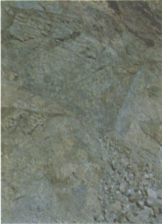
Fig. C-5 - A 3-d-wedge slide where the bounding planes did not daylight into the slope face, requiring crushing at the bottom point of the wedge to permit movement.
