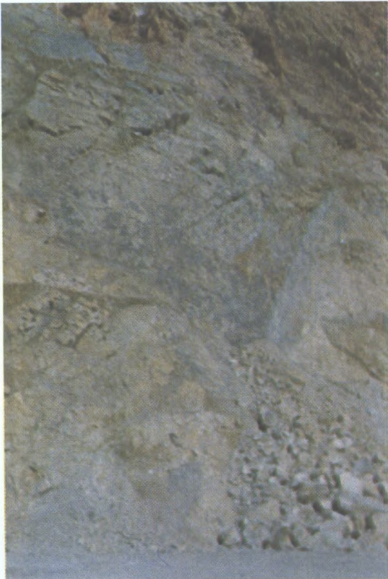
Fig. 33 - A minor slide caused by wedge geometry. The wedge, which was bounded by three planes that did not daylight into the slope, crushed at its bottom point.
