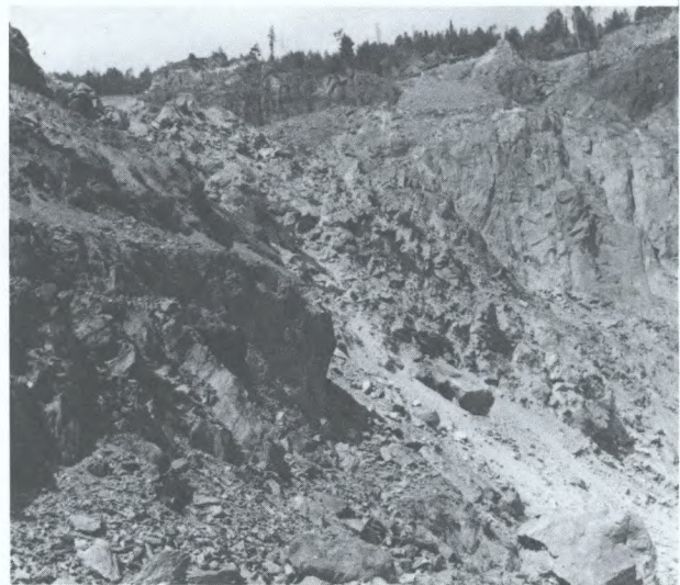
Fig. 32 - Slope instability caused by toe crushing. A slope 445 ft (136 m) high at 51° failed in a manner suggesting initiation was by toe shearing followed by a general breakdown of the rock mass.
