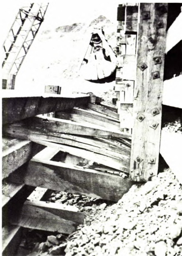
Fig 50 - Structural damage to members of buttress at IOC due to settlement.
