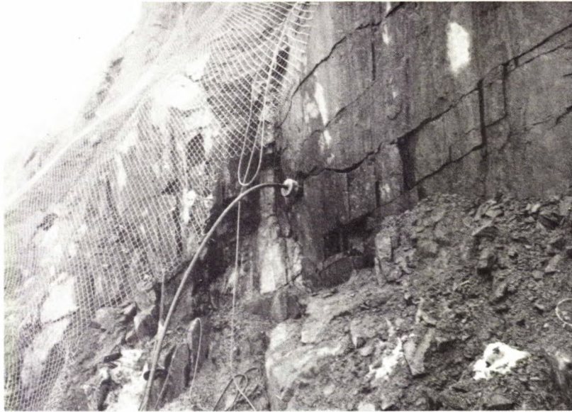
Fig B-9 - The rock at the surface of the anchor is sufficiently competent for the block to bear directly on the rock. The anchor hole has been over-reamed to allow this.
