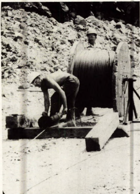
Fig B-6 - Cutting pre-stressing strand prior to laying out an anchor. Cutting is done with a carborundum wheel.
