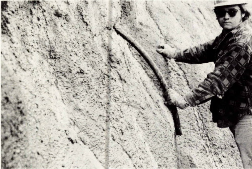
Fig C-11 - Provision must be made for draining shotcrete. Here a drainage tube has been wedged in a crack in the concrete face before spraying.
