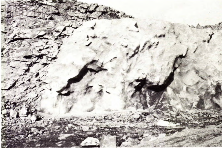
Fig C-10 - A view of shotcreting showing the contact between sprayed and unsprayed sections.
