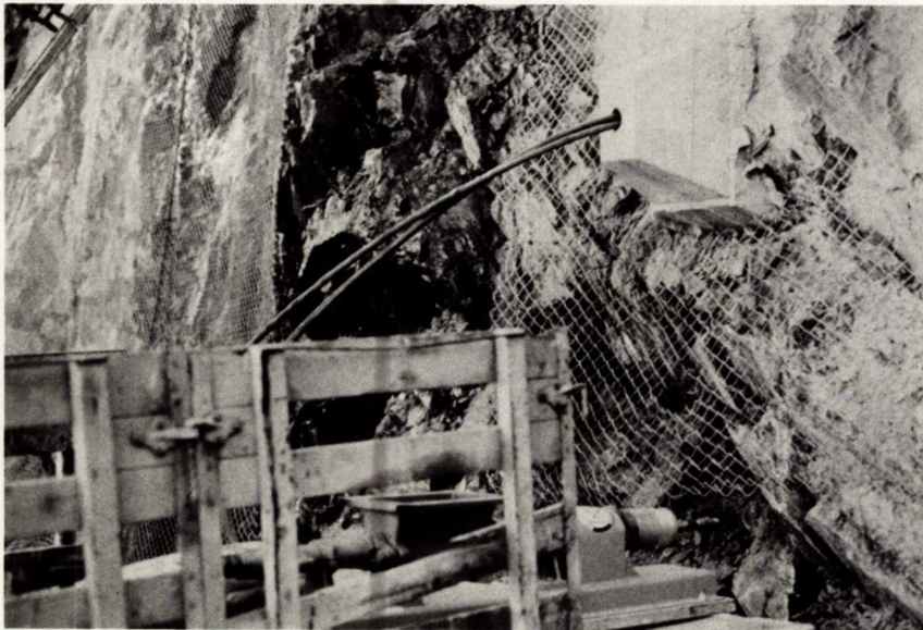
Fig E-10 - A completed surface anchorage showing the concrete bearing block. A grout tube can be seen emerging next to the anchor cable.
