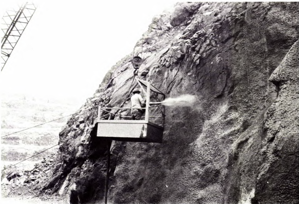
Fig C-7 - Top: General view of a spraying operation at an open pit mine. The drill rig in the centre is being used to supply compressed air; the shotcreting machine is behind the rig. Bottom: Close-up of the spraying platform.
