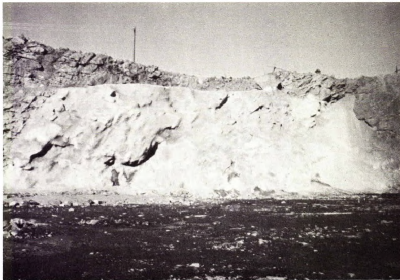
Fig C-15 - Top: A slope before spraying. Bottom: Centre of the same slope after shotcreting. Location of the sprayed section can be judged from the pole supporting a power line behind the slope.
