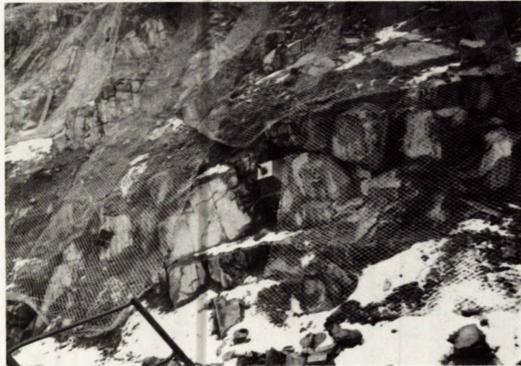
Fig 18 - Mesh used as protection against loose rock. A concrete bearing block for a rock anchor is seen in the centre of picture.
