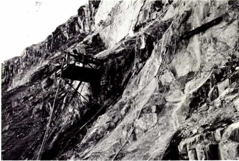
Fig E-7 - Wire mesh used for control of loose rock during anchor installation.
