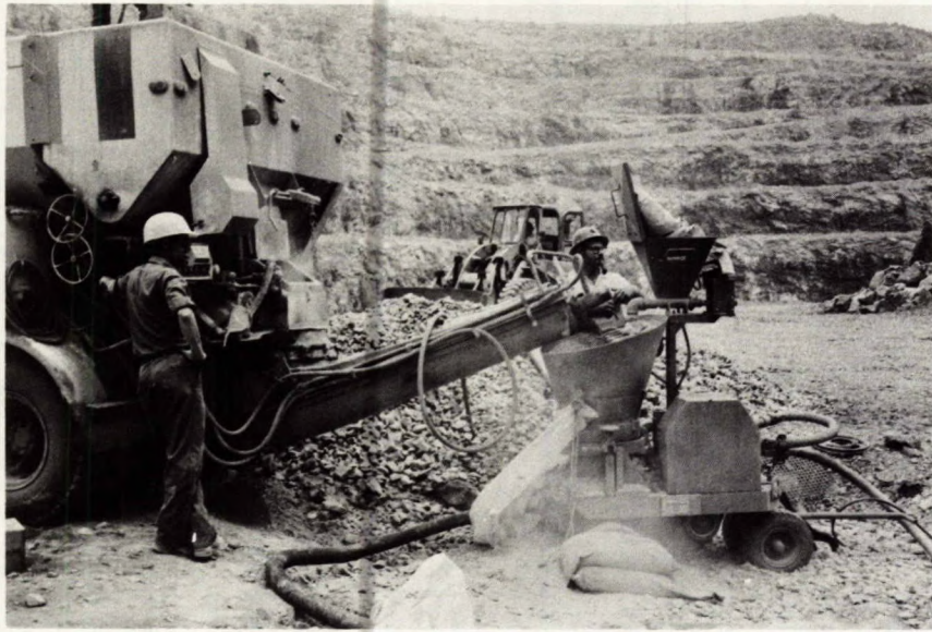
Fig C-5 - The Icoma Shotcrete Machine being fed by a cement mobile batching truck.
