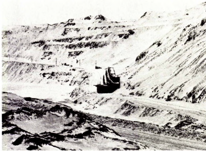
Fig 16 - A buttress used to stabilize a slope in a large Canadian iron ore mine.
