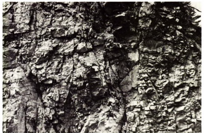
Fig 44 - Backbreak and loose face rock on pre-split surface in intensely fractured rock.
