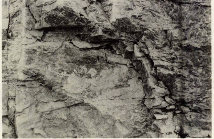
Fig 47 - Backbreak and loose face rock due to undercut jointing almost parallel to pre-split line.
