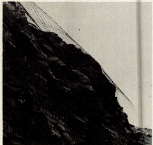
Fig 33 - A field experiment using rock anchors and mesh for mechanical support of part of a wall.
