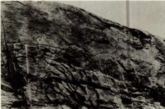
Fig 46 - Pre-split surface corresponds to major jointing parallel to rock face.
