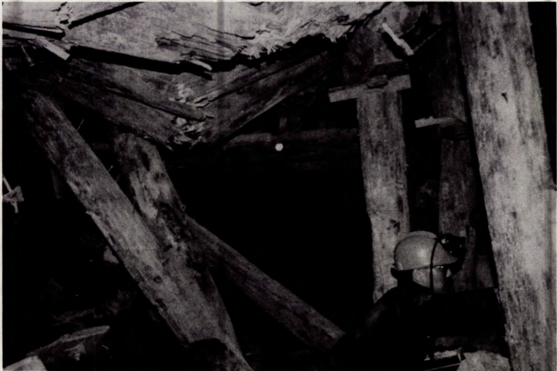
Damage to wooden posts and beams at Macassa Mine.
