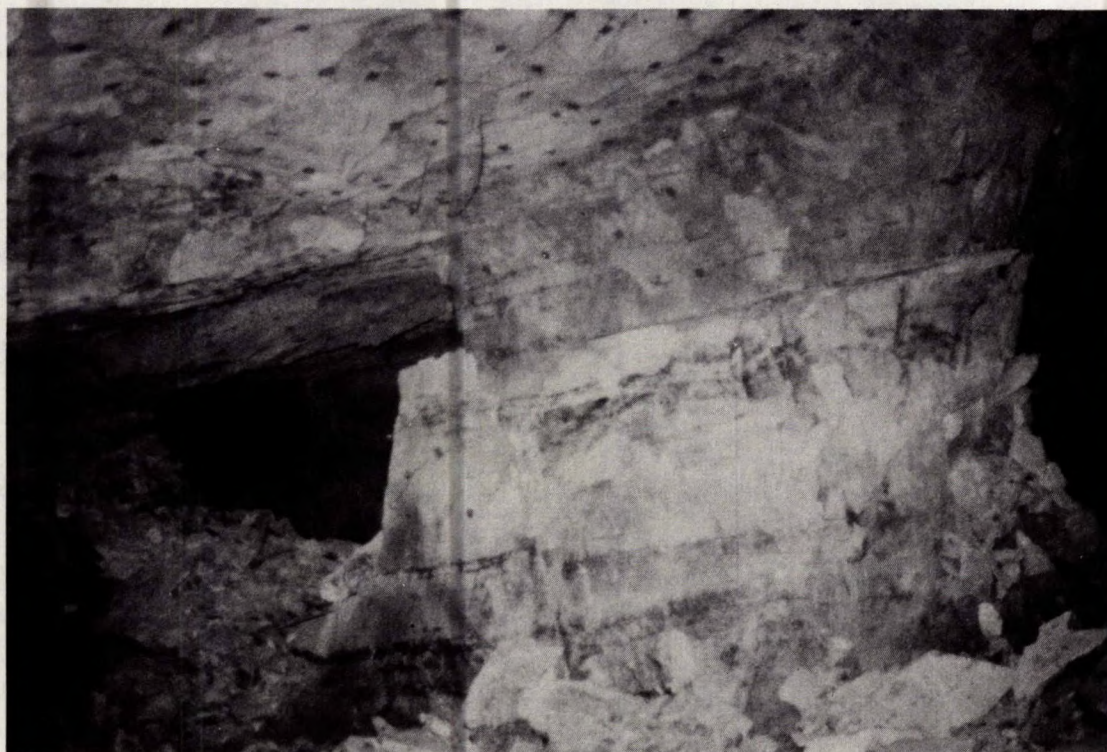
Slippage along a bedding plane in a pillar at Denison Mine.
