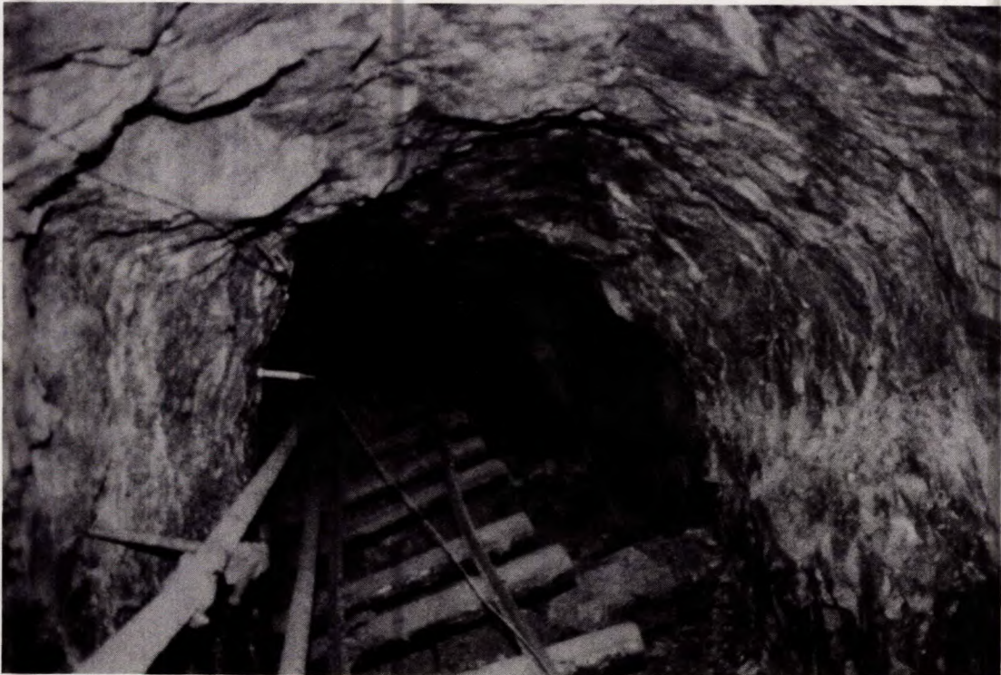
Floor heave due to rockbursts at Campbell Mine.
