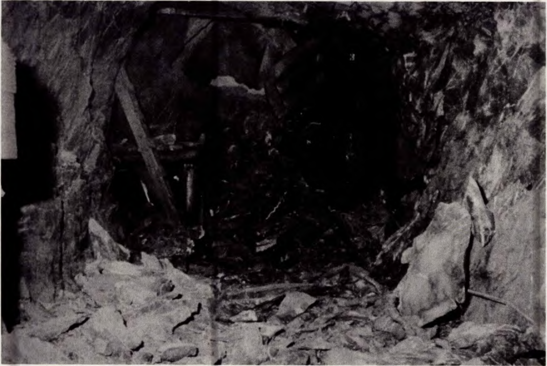
Blocked drift at edge of rockburst area at Campbell Mine.
