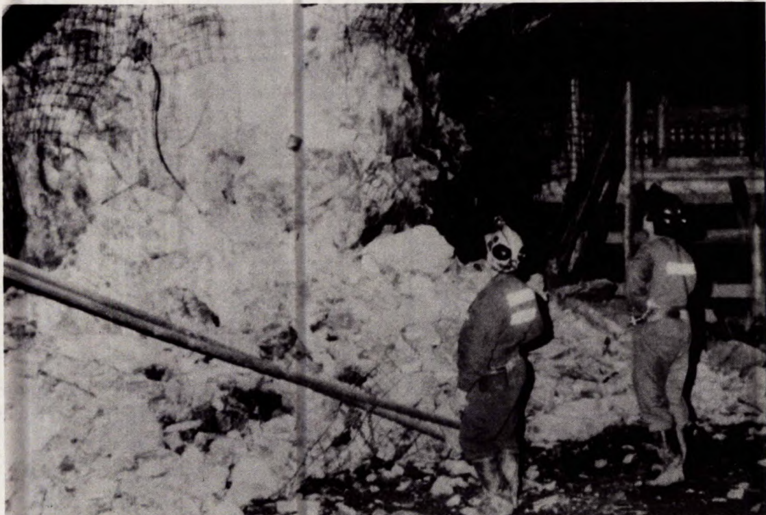
Damage to a ramp at Strathcona Mine prior to initiating destress blasting.
