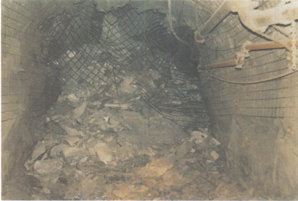
Damage to a drift on the 6600 level of Creighton Mine, caused by a 3.6 Mn rockburst about 25 m away.
