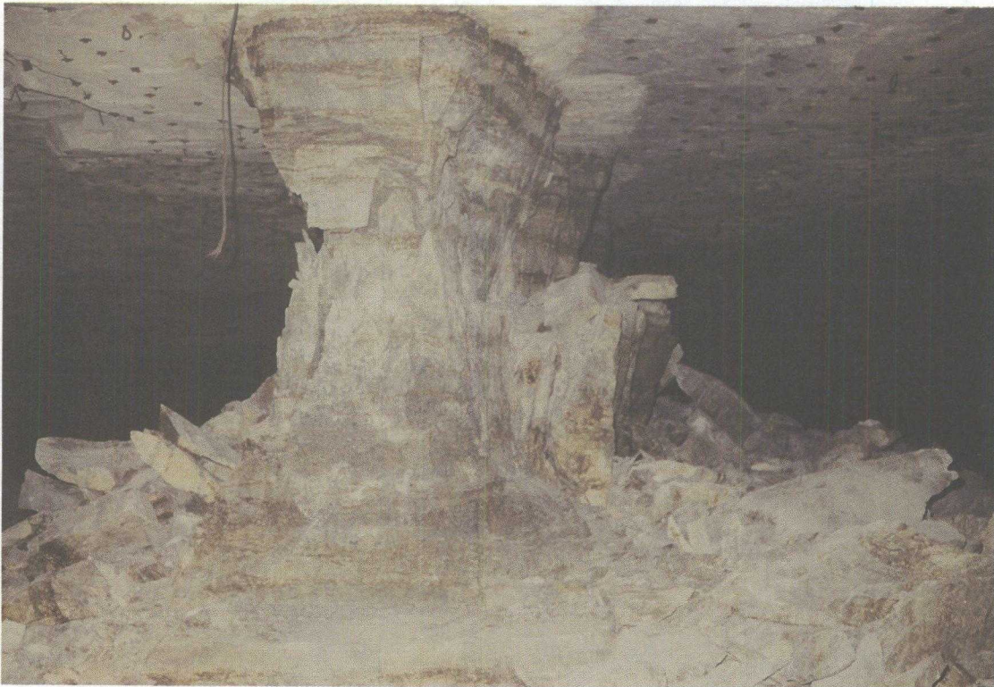
Spalling of a rib pillar in the rockburst area on the east side of Denison Mine.
