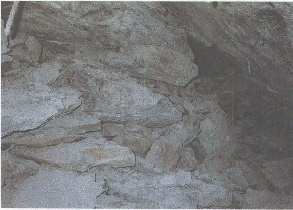
More than 800 tonnes of rock displaced because of two small (2.0 Mn) rockbursts in an isolated haulage drift at Strathcona Mine.
