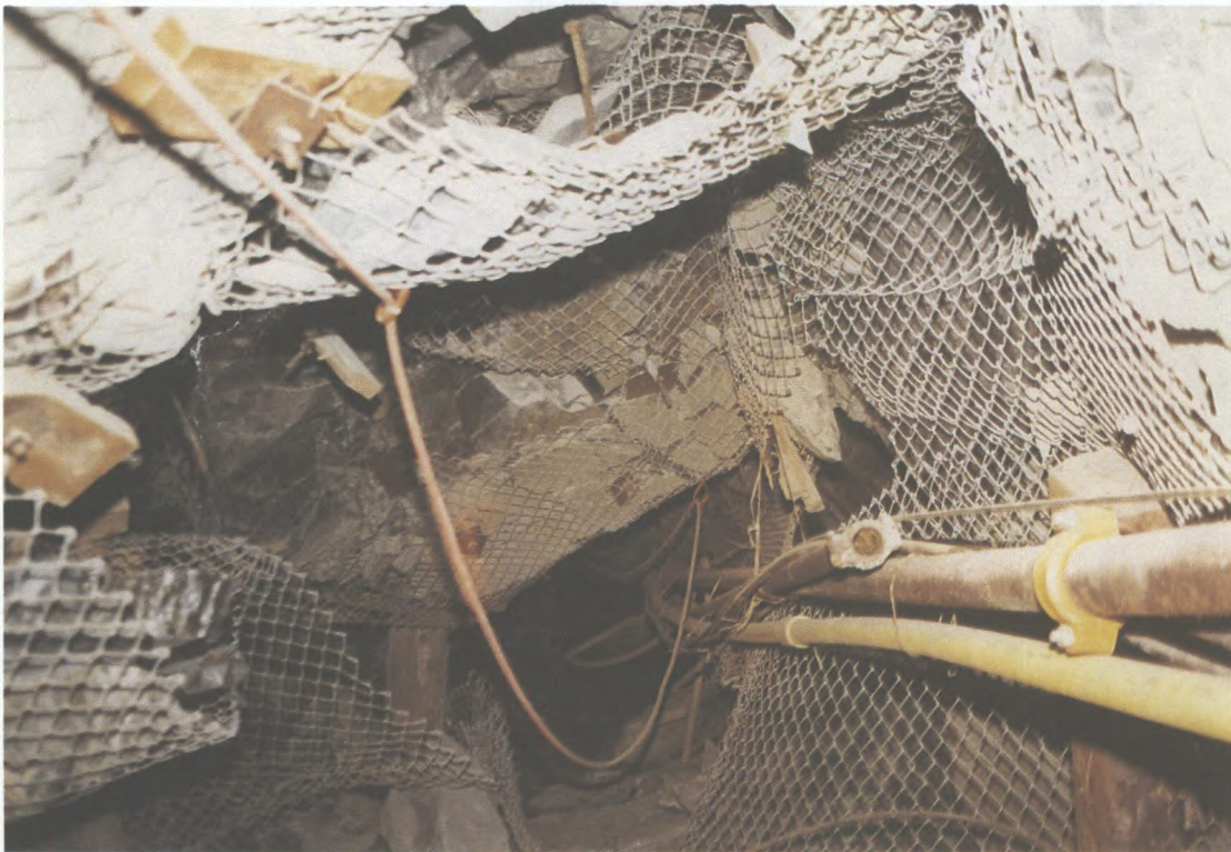
Damage caused by a 3.1 Mn rockburst at the Macassa Mine. Bolts and chain-link mesh prevented completed closure of the drift.
