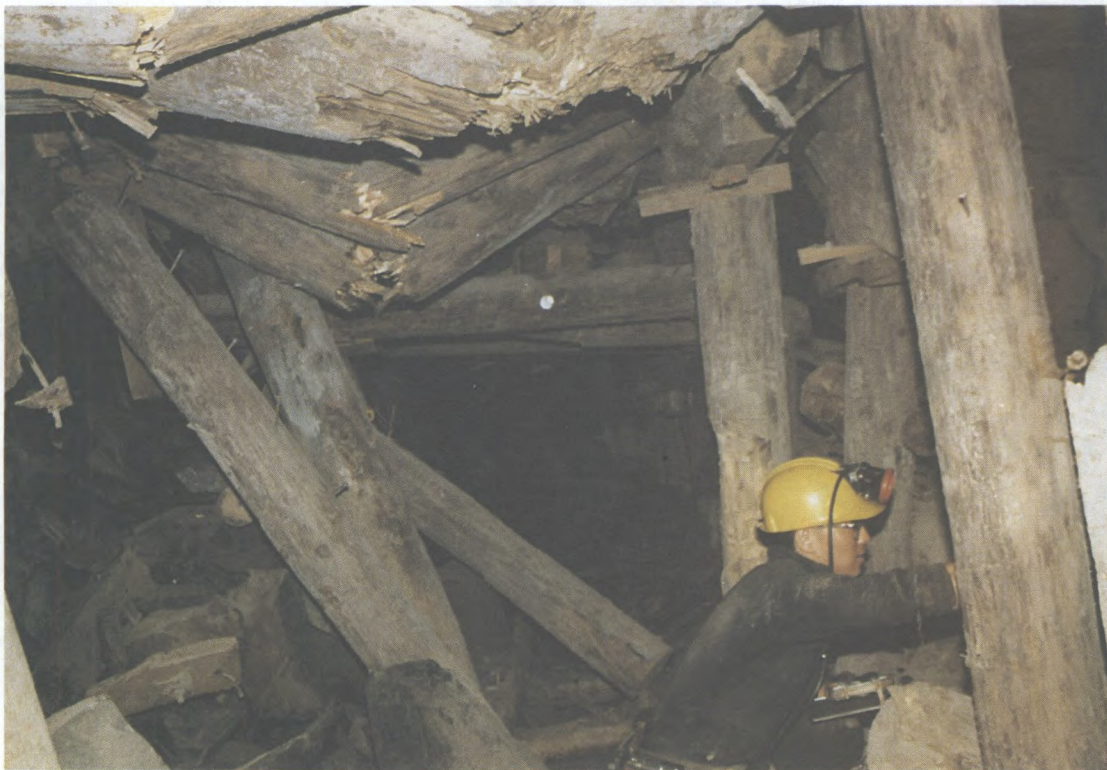
Rockburst damage to a drift supported by timber posts and beams at the Macassa Mine.
