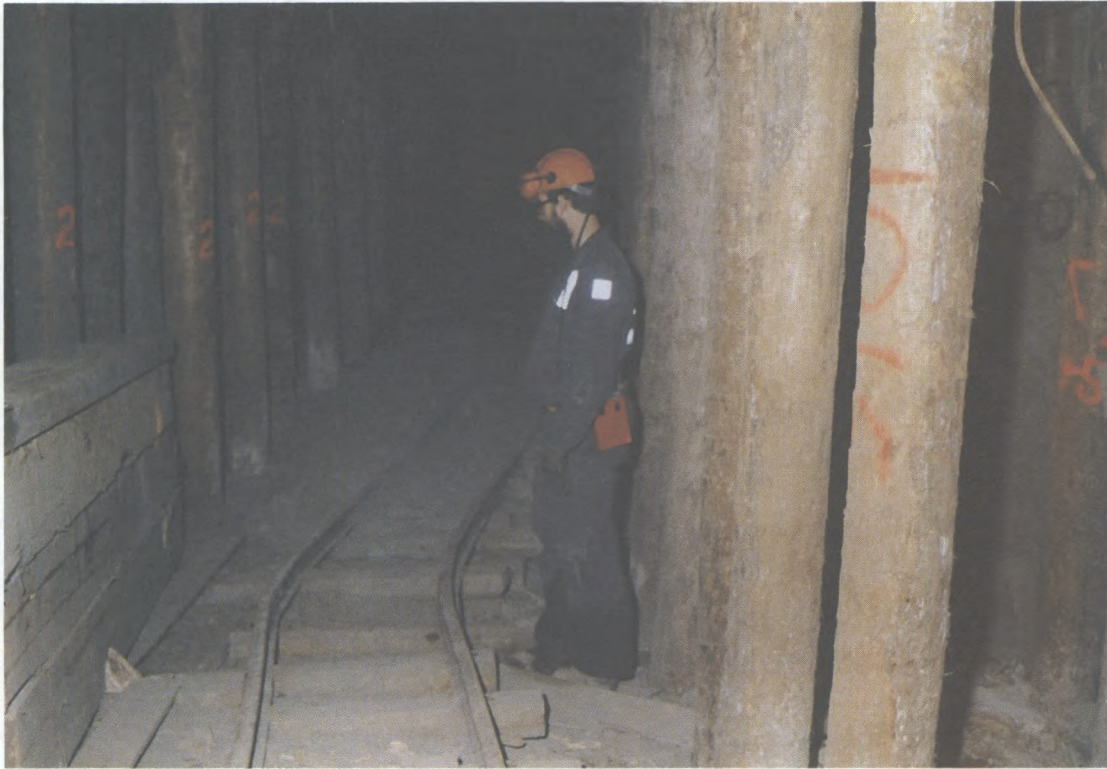
Displacement of the track caused by fault slippage at Falconbridge's No. 5 shaft.
