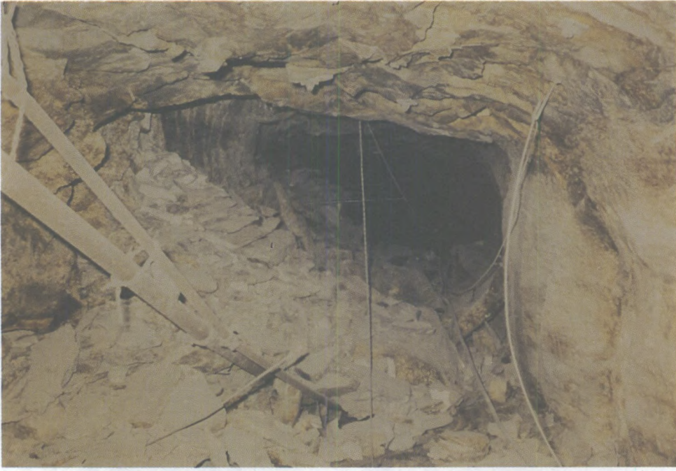
Damage to a sill drift at the Quirke Mine.
