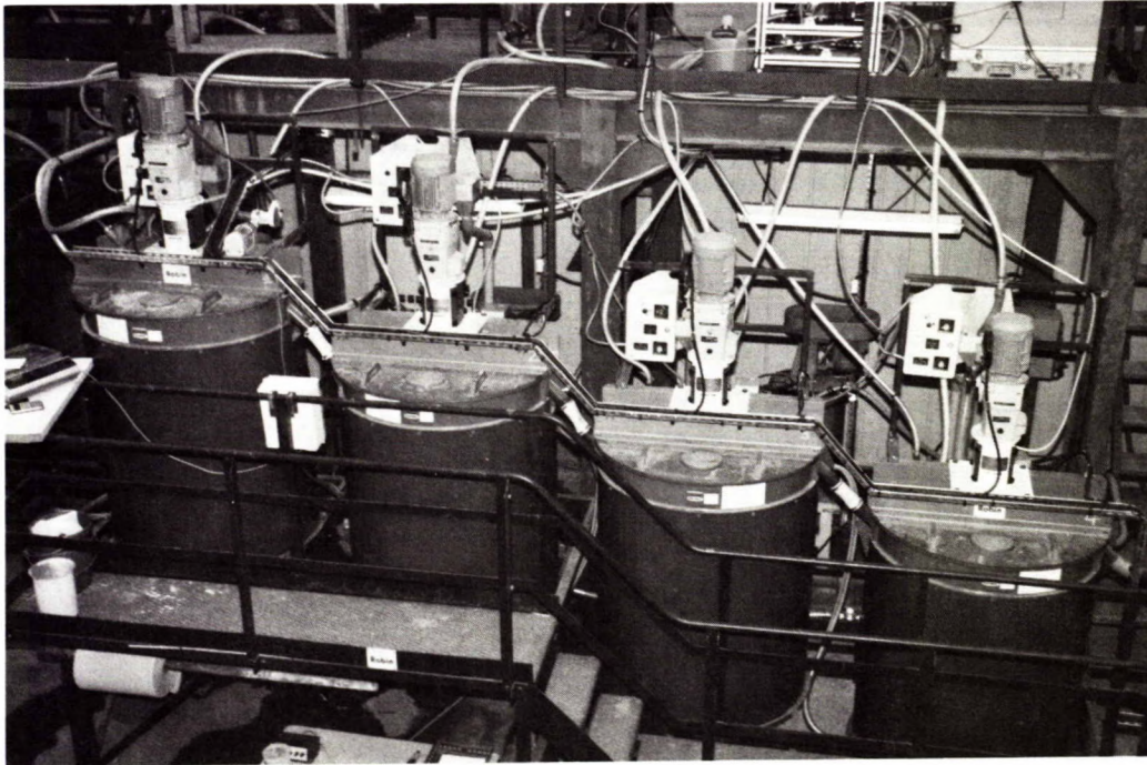
Photo 1 View of the cascade of reactors of the 3.2 m 3 unit.
