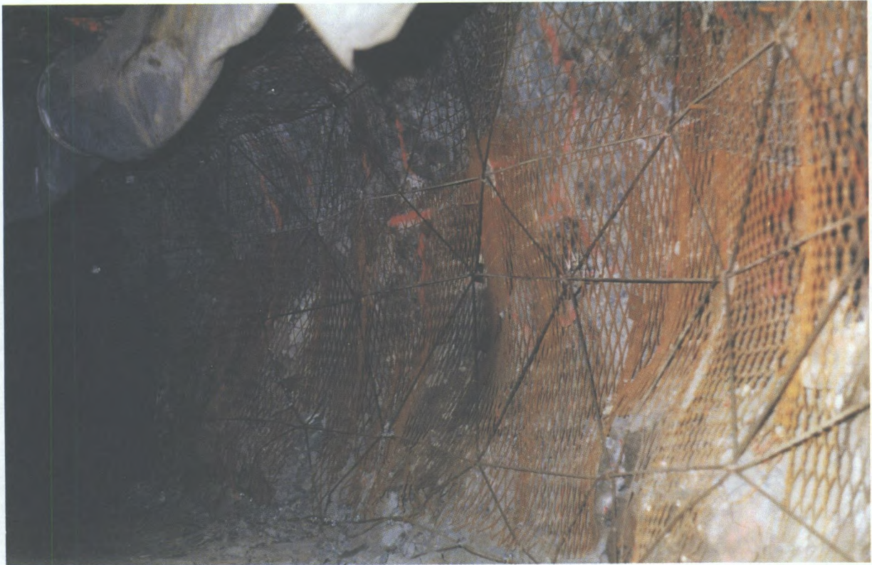
Lacing installation at Strathcona Mine. Subsequently, a rockburst of 3.0 M_N occurred 40 m away without damaging the laced section, although an adjacent conventionally supported area collapsed.
