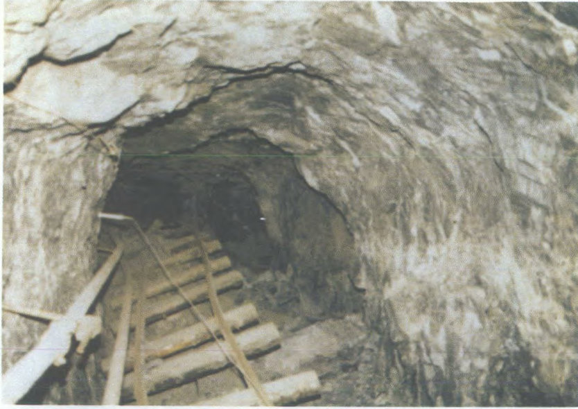
Rockbursts in crown pillar in F ore zone, Campbell Mine. Track has heaved at least 1 m.
