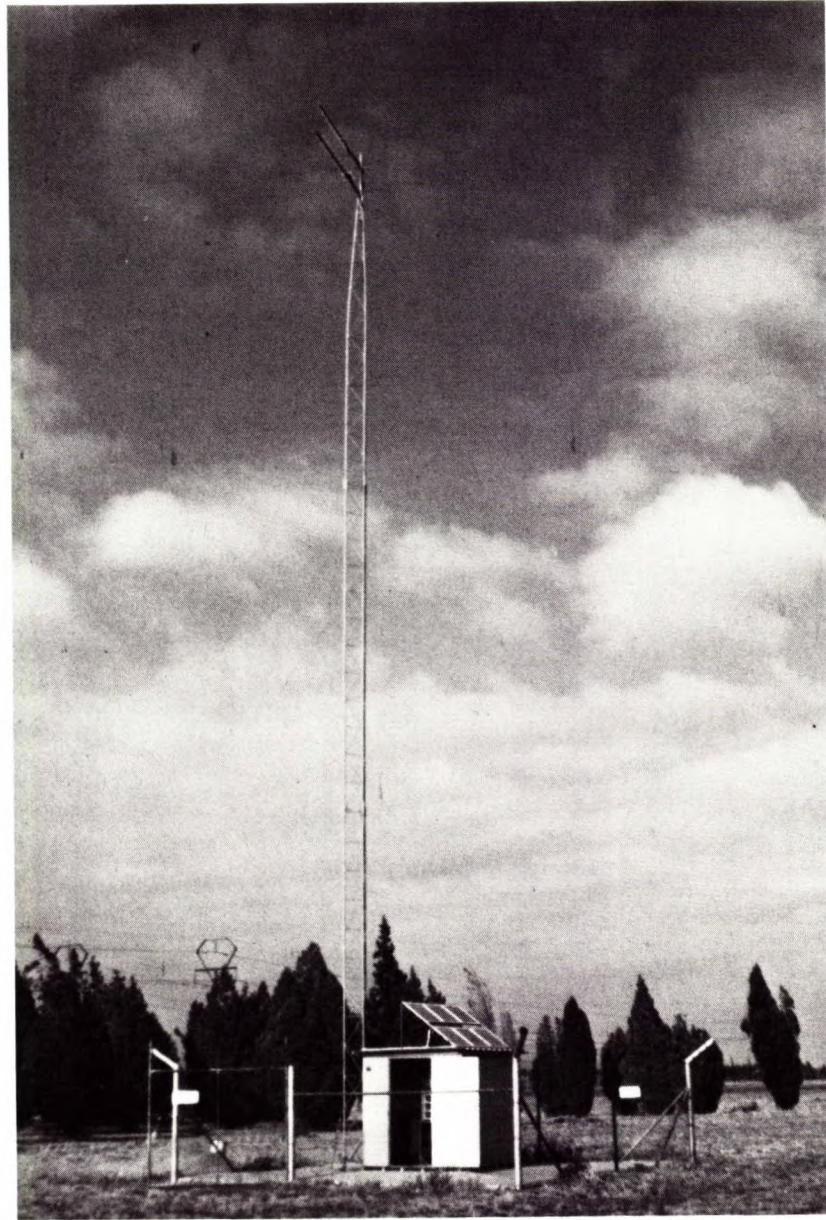
Figure 11. Surface field site for microseismic network. Data transmitted by radio. The complex electronic equipment is powered by solar electricity. (Anglo American Corporation)
