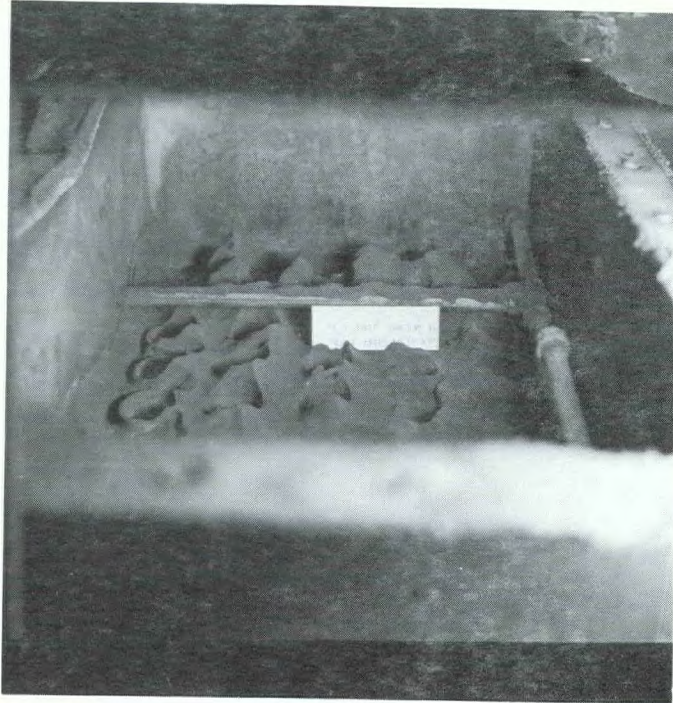
FIGURE 1f Main air heater tube sheet second pass up to 2 - 3 inches of powder.
