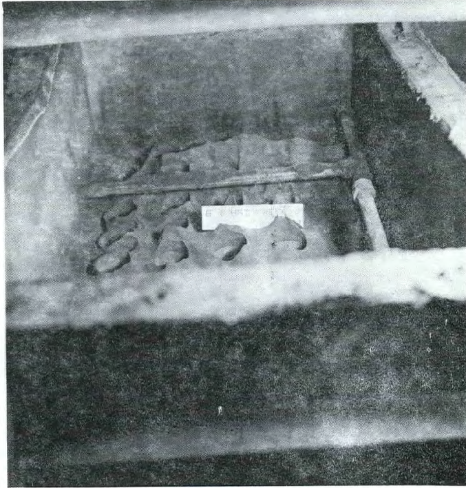
FIGURE 1f Main air heater tube sheet second pass up to 2 - 3 inches of powder.
