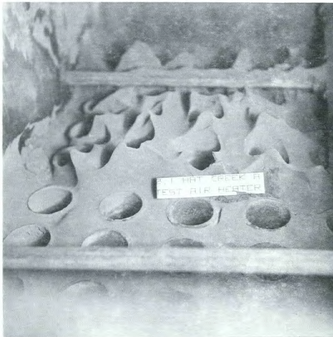
FIGURE 1i Main air heater tube sheet second pass up to 2 - 3 inches of powder
