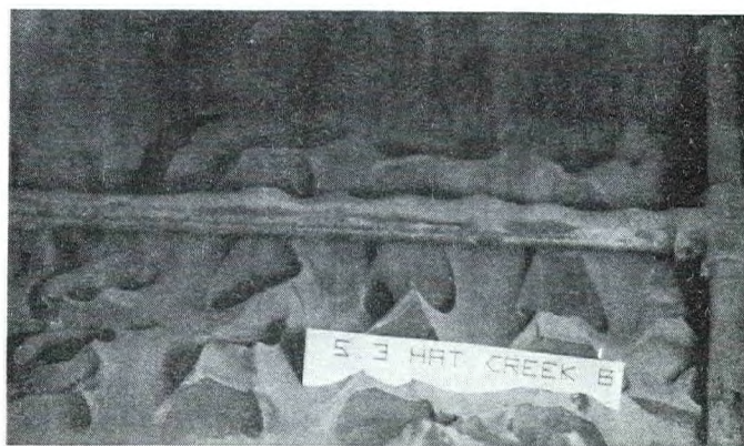
FIGURE 1b Main air heater tube sheet second pass up to 2 - 3 inches powder.
