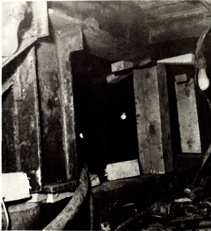
Figure 36. A greased timber skid resting on the cutterhead canopy; steel beams forming a cage support are shown at the top of the photograph.
