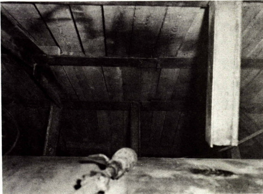
Figure 33. Over-mining support above the top of the cutterhead canopy.
