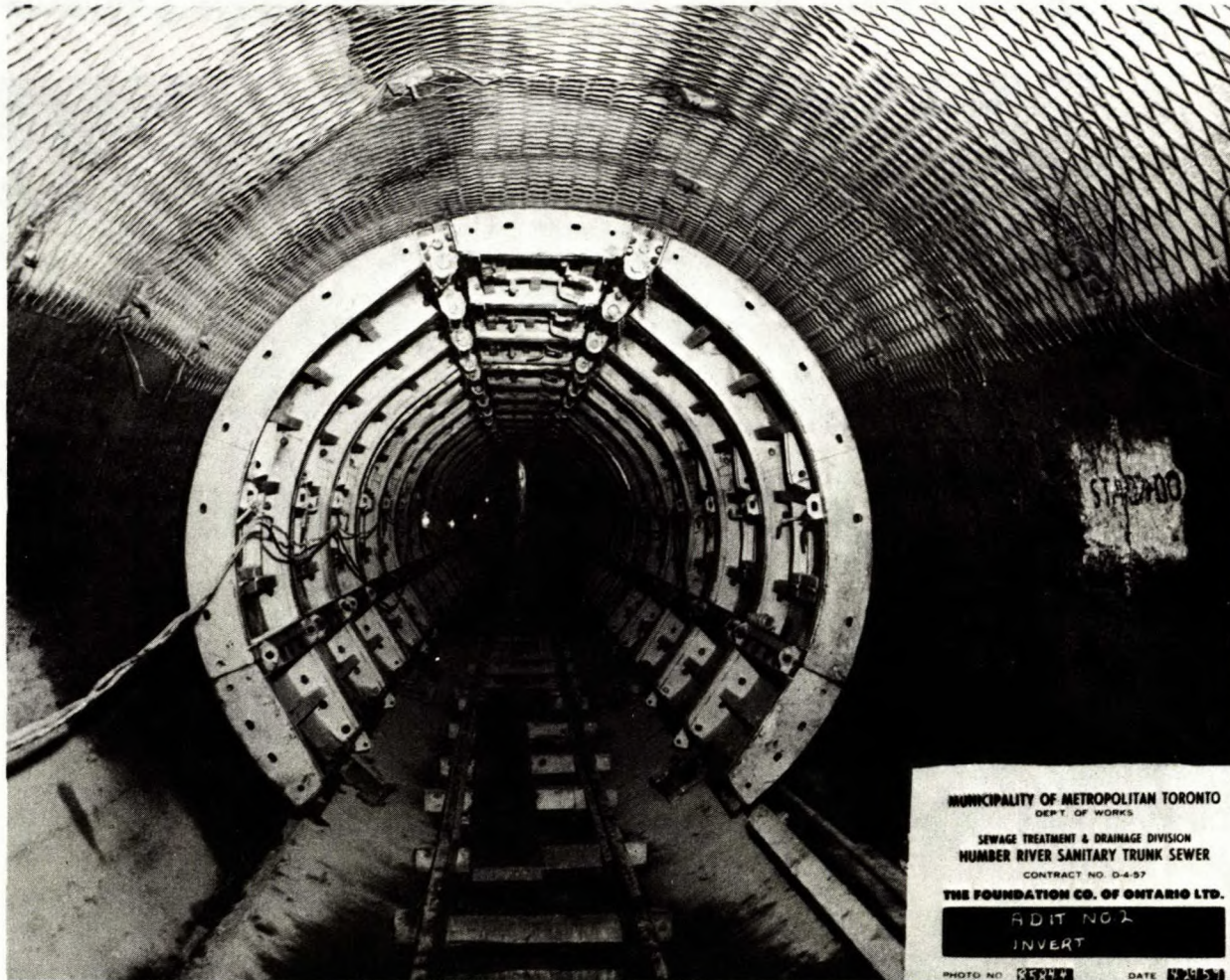
Figure 11. View of collapsible steel forms in place to receive concrete for construction of concrete lining. Note concrete section already in place in tunnel invert and carrier for moving the forms in background.
