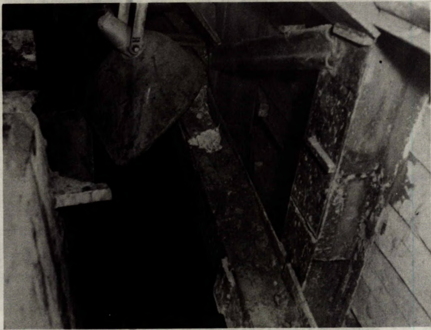
Figure 34. A hand-mining area in front of the cutterhead, with the front of the cutterhead shown at left.
