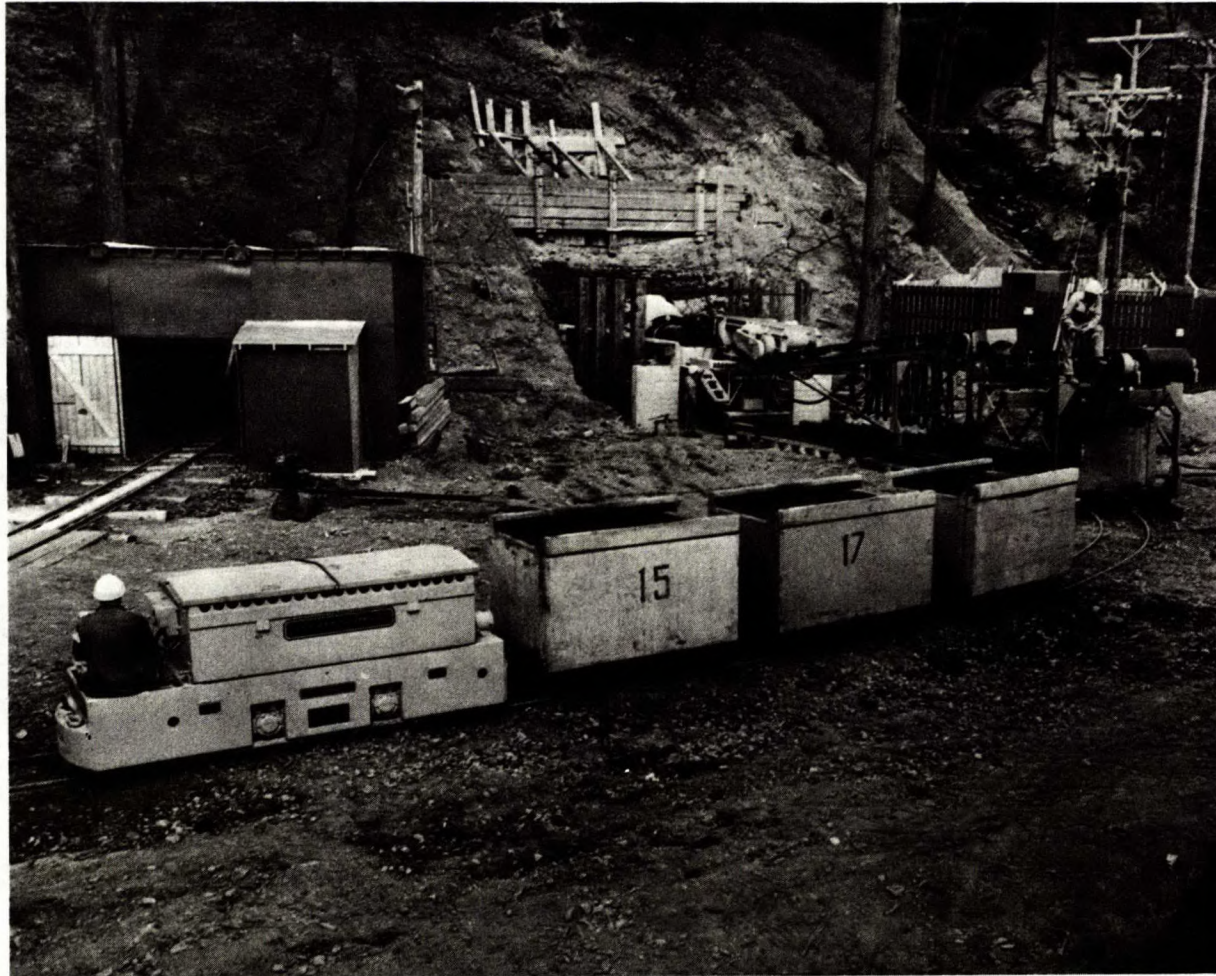
Figure 9. General arrangement of Foundation Humber boring machine with trailing conveyors and muck train in position at commencement of boring operations.
