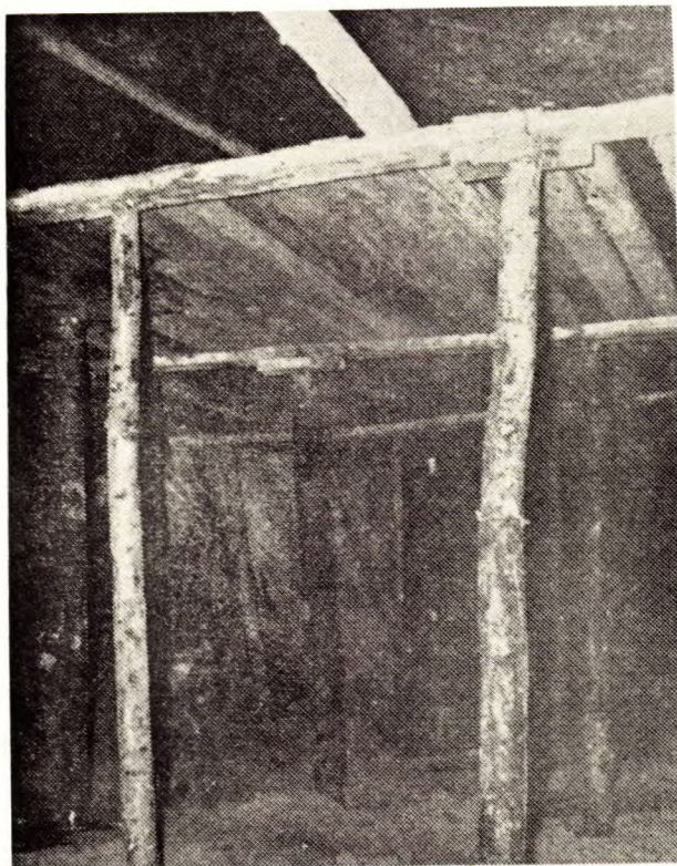
Figure 2. Elevated stope floor carrying fill pipes.
