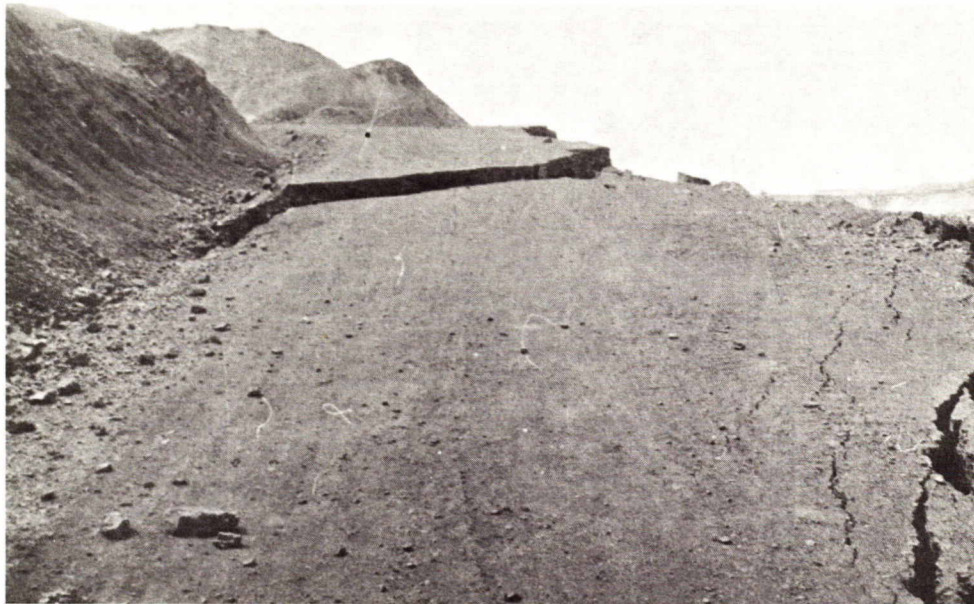
Figure 9. Two-foot-wide crack at the crest of the second slide, July, 1963.
