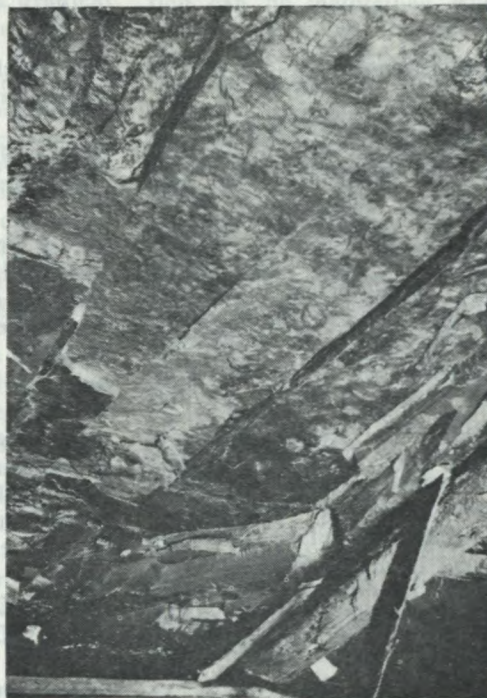
Figure 1.—Typical joint system in roof shale, causing a minor fall. Such falls near the face aggravate the installation of bolts. (photo courtesy of D. K. Norris)
