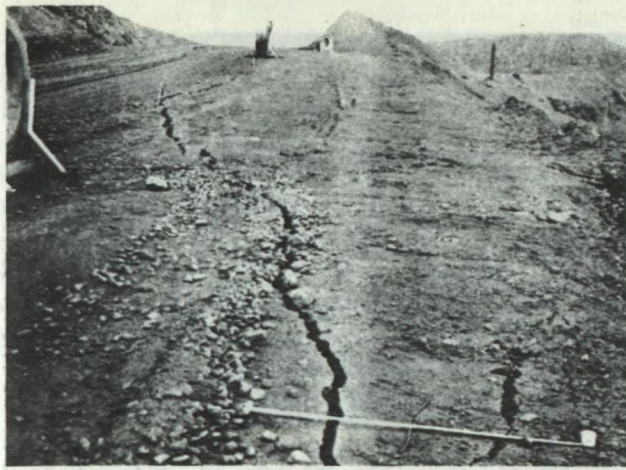
Fig. 10—Tension cracks developing at the top of the slope of slide No. 2 in altered slate and quartzite.
