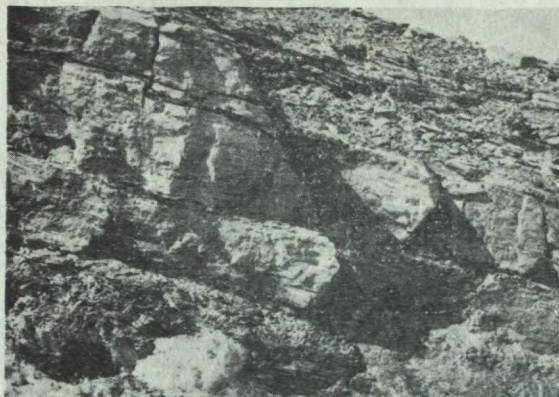
FIG. 2—Geological structures favouring plane shear failure.
