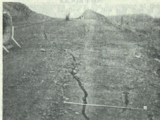
FIG. 10—Tension cracks appearing in the crest of the wall in Fig. 8, July 1961.
