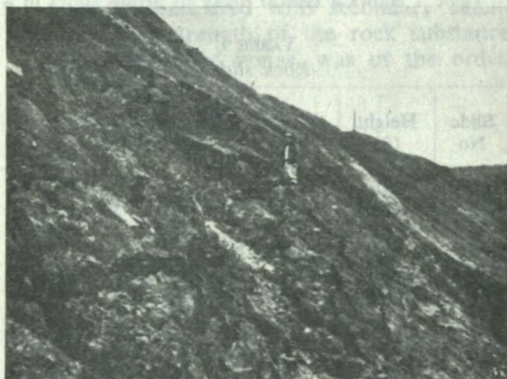
FIG. 11—A small slide in the same wall adjacent to the main slide zone, July 1961.
