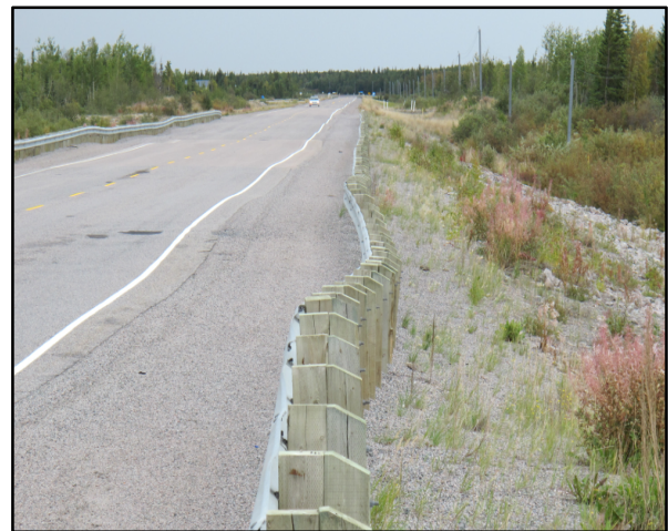
Subsidence and slope movement on the new NWT Highway 3 due to ground settlement and thawing of permafrost beneath the embankment. Photo by S. Wolfe.
