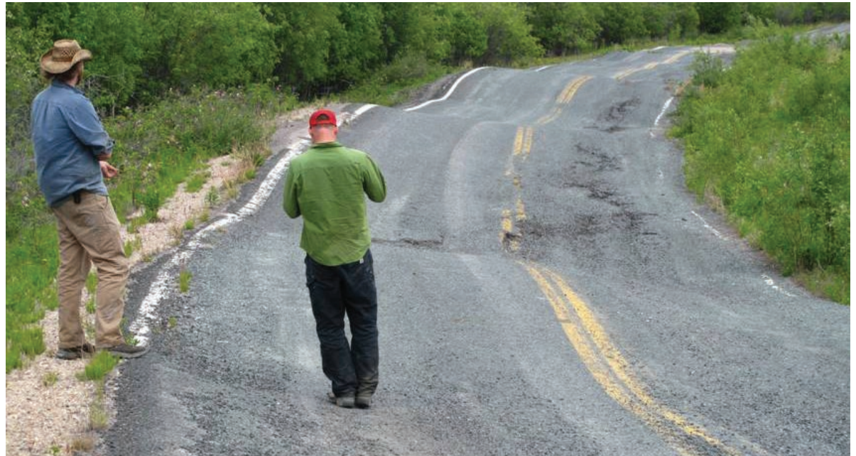
Abandoned section of NWT highway 4, east of Yellowknife, being examined for damage caused by permafrost thaw. Source: Natural Resources Canada
