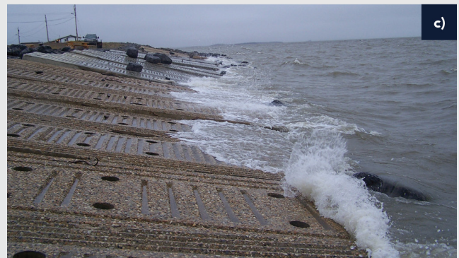
FIGURE 23: Various types of shore-protection measures include a) sandbags put in place in 1987, b) stone boulders (rip-rap) first used in 1997, and c) monolithic concrete slabs that were installed in 1998. Photos a) and b) courtesy of S. Solomon, and photo c) courtesy of G. Manson.
