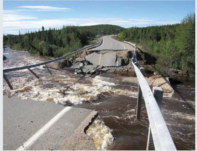
FIGURE 4: Washout of highway and bridge near Port Rexton, NL. Photo courtesy of Fire and Emergency Services, Newfoundland and Labrador.
