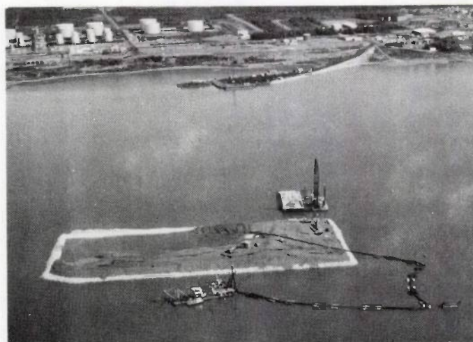
Construction of Rampart Island, showing dredging and in-filling of the initial rock rim.
