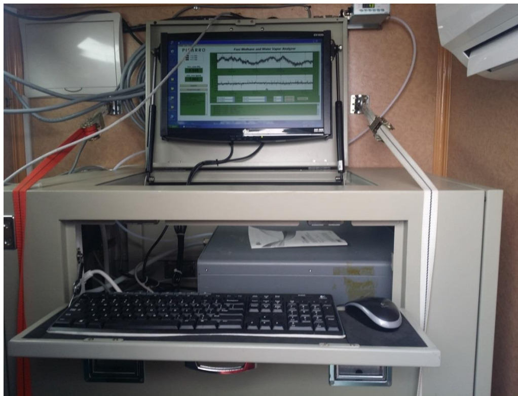
Figure 11.3 - Close path gas analyzer (CRDS) in the CRDS container.
