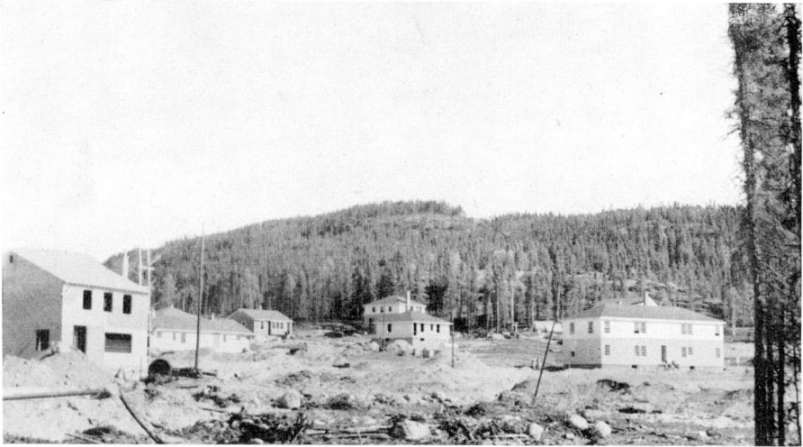
A. Part of staff quarters (under construction), Eldorado Mining and Refining (1944) Limited, Beaverlodge Lake, Saskatchewan. (4-3, 1951.) (Page 68.)
