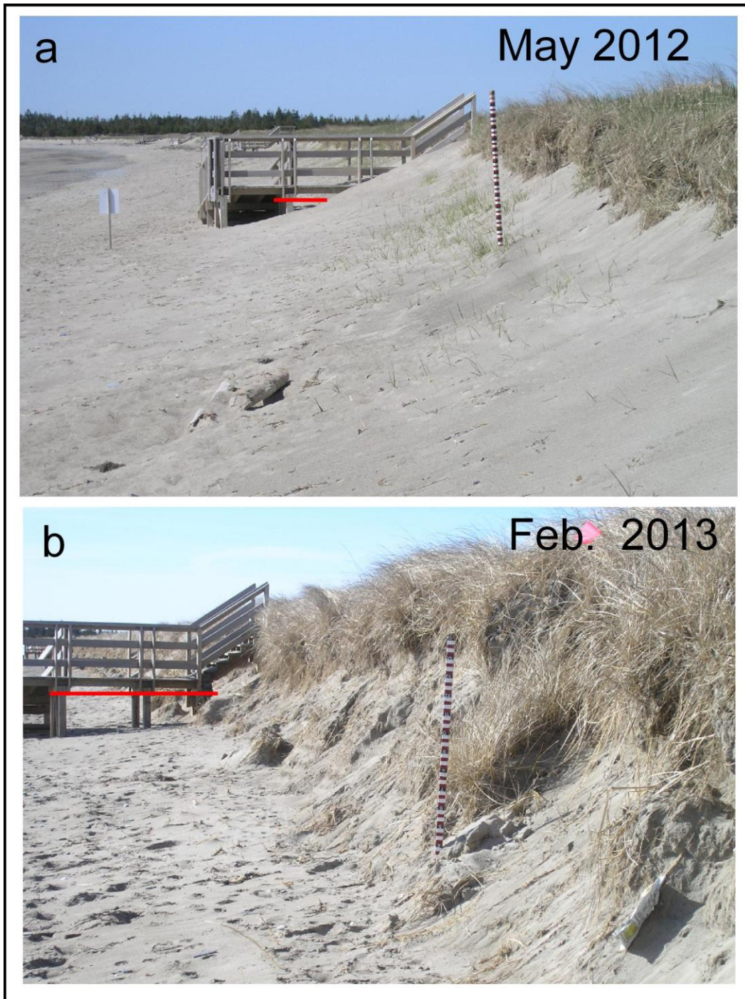
Figure 23. Martinique Beach: Repetitive photos taken at line 3 on (a) May 2012 and (b) February 2013 illustrate the loss (marked by red line) of a wide sand ramp which had heralded dune stability and growth in 2012. Waves during the February 9, 2013 storm scoured the upper beach and trimmed the foredune but were insufficient to damage beach access stairs. The wooden graduated pole marks the location of line 3 and provides a scale -it is graduated in 2 cm intervals.
