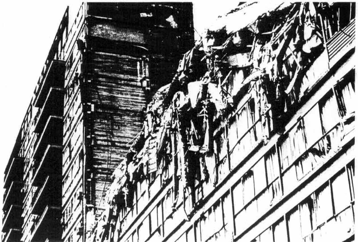
Fig. 6.13a and 6.13b Collapse of Top Six Storeys of Continental Hotel
