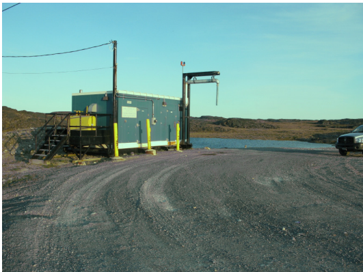
Water pumping station and truck loading station at the actual supply lake.
