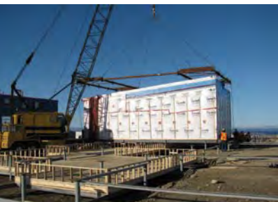
Ground preparation at the PCSP facility for installation of modules (Resolute, Nunavut).
