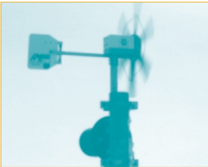
▲ This remote radio repeater in Kananaskis, Alberta uses solar energy to produce electricity in addition to wind. (Photo courtesy of Nor'wester Energy Systems Ltd.)
