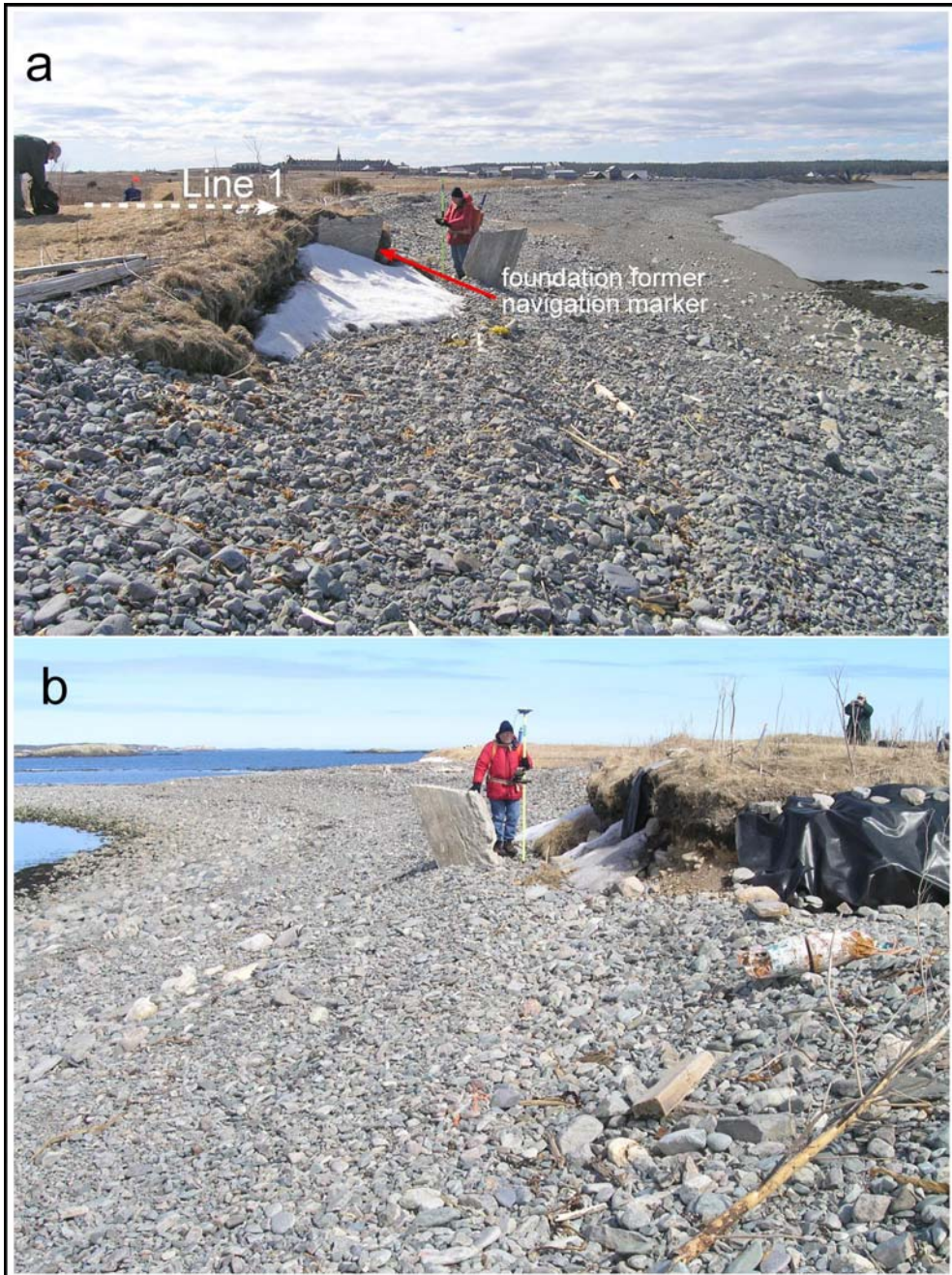
Figure 1540-2. Views alongshore of beach and shore bank conditions at site 1540 in March 2011. (a) shows recent beach sediment build-up against the shore bank that was eroded and a large slab of concrete broke away from the foundation and (b) shows the human burial site (geofabric cover) just north of the concrete foundation. Survey line 1 is at person in background.
