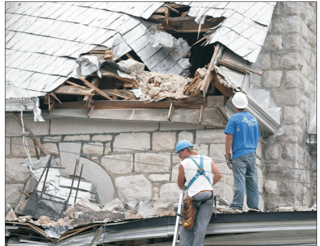
Damage to a church from a falling chimney in Gracefield, QC (Adrian Wyld, The Canadian Press)
