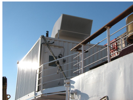
Figure 5.17 Hurricane Compressor, (HC #1), fitted to the starboard side of LSSL.
