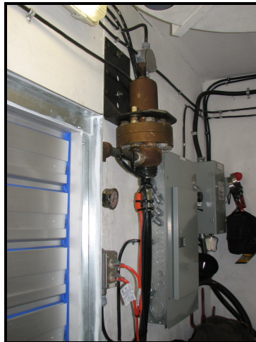
Figure 5.13 6000 SCFM back pressure valve as fitted to HC #1 container bulkhead.
