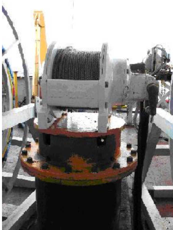
Figure 5.6 Centre tugger winch mounted on the forward bollard, amidships, used for tow cable and bundle deployment and recovery.
