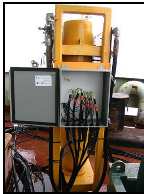
Figure 5.14 Electrical junction box for starboard sled showing internal wiring.
