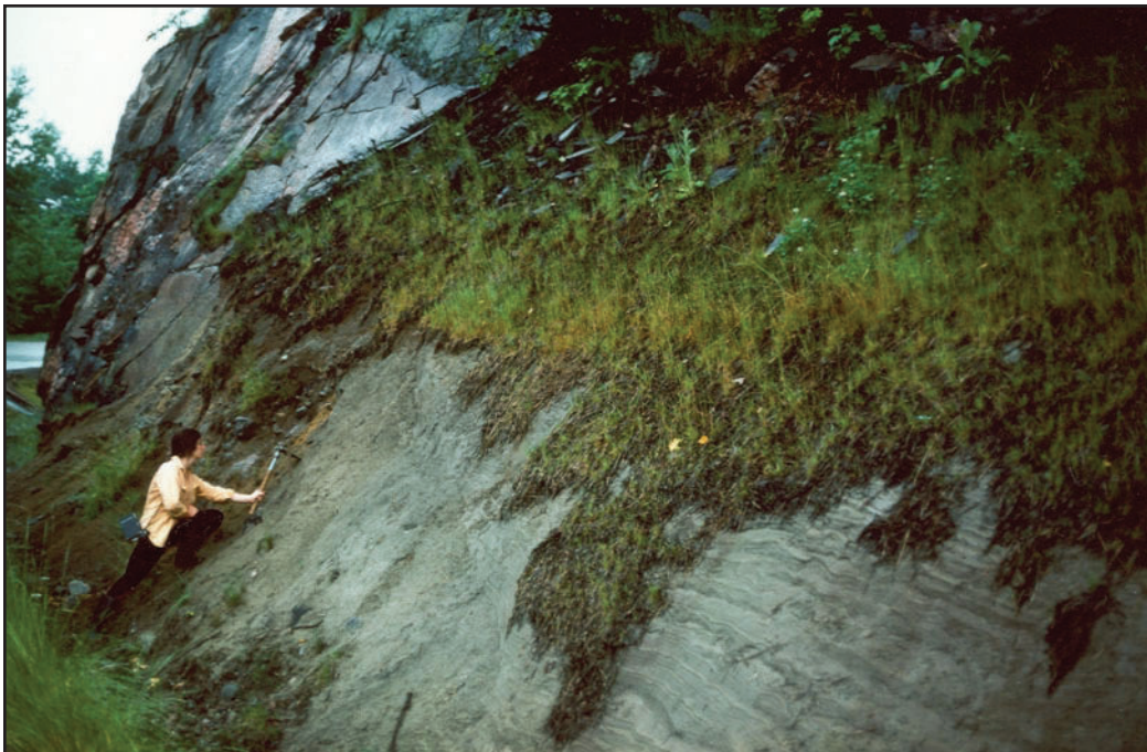
Figure 5-3. Road cut exposure of till (in the vicinity of sampler) overlain by glaciolacustrine finely bedded fine sand and silt (bottom right). Both types of sediment were deposited over rugged Precambrian shield bedrock in south-central Ontario.
