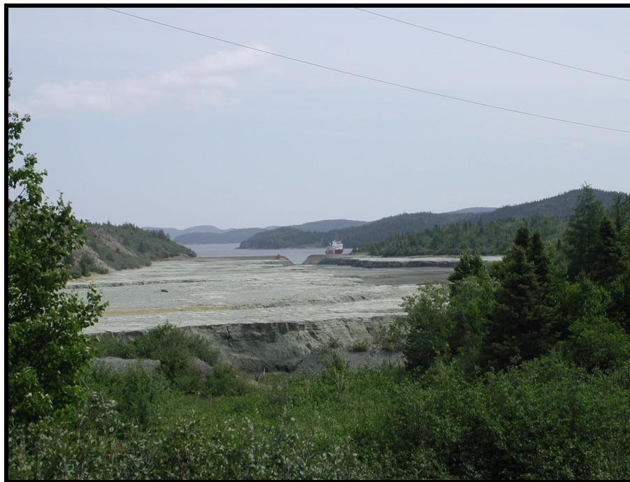
Breached tailings impoundment at the Little Bay Mine with CCGS Matthew in background.
