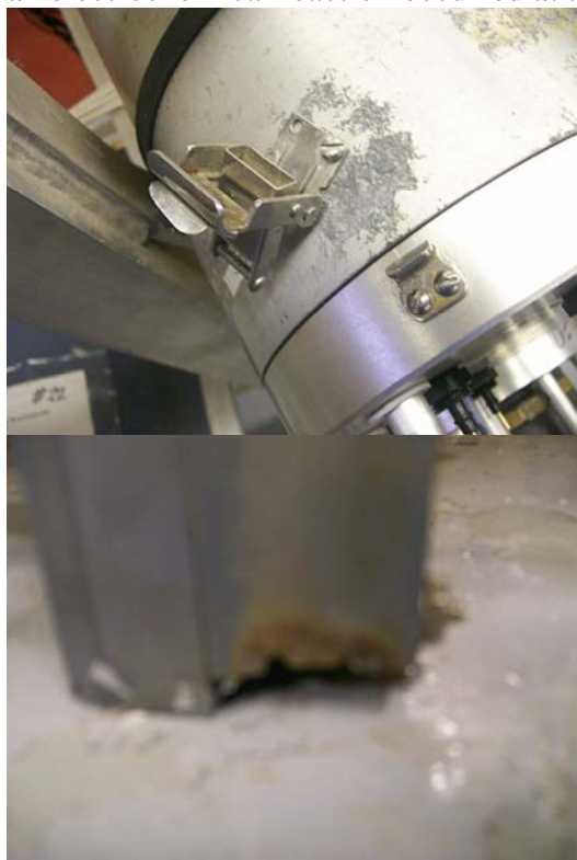
Figure 9. Broken screw on the cylinder latch of OBS E after it was hit by a wave.
