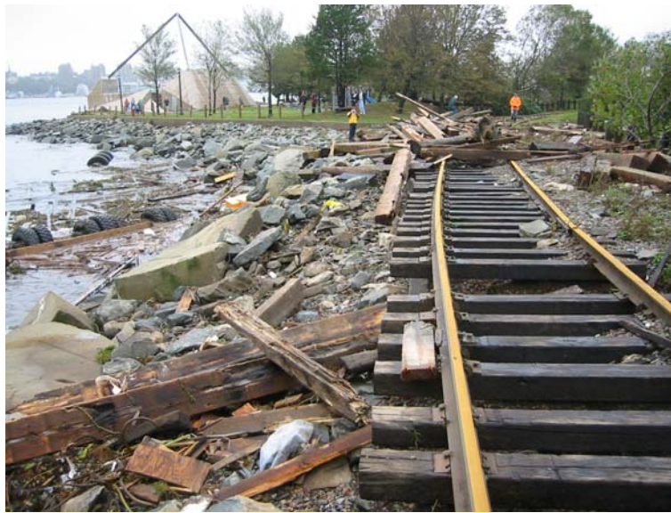
Fig. 4. Debris deposited on and beneath undercut CN rail line at Dartmouth Point on the morning after Hurricane Juan. Runup here was 1.64 m above the highest water level recorded at the Halifax tide gauge across the harbour. Note that water level remains unusually high at the time of photography. Photo: DLF/GSC, 2003-09-29.
