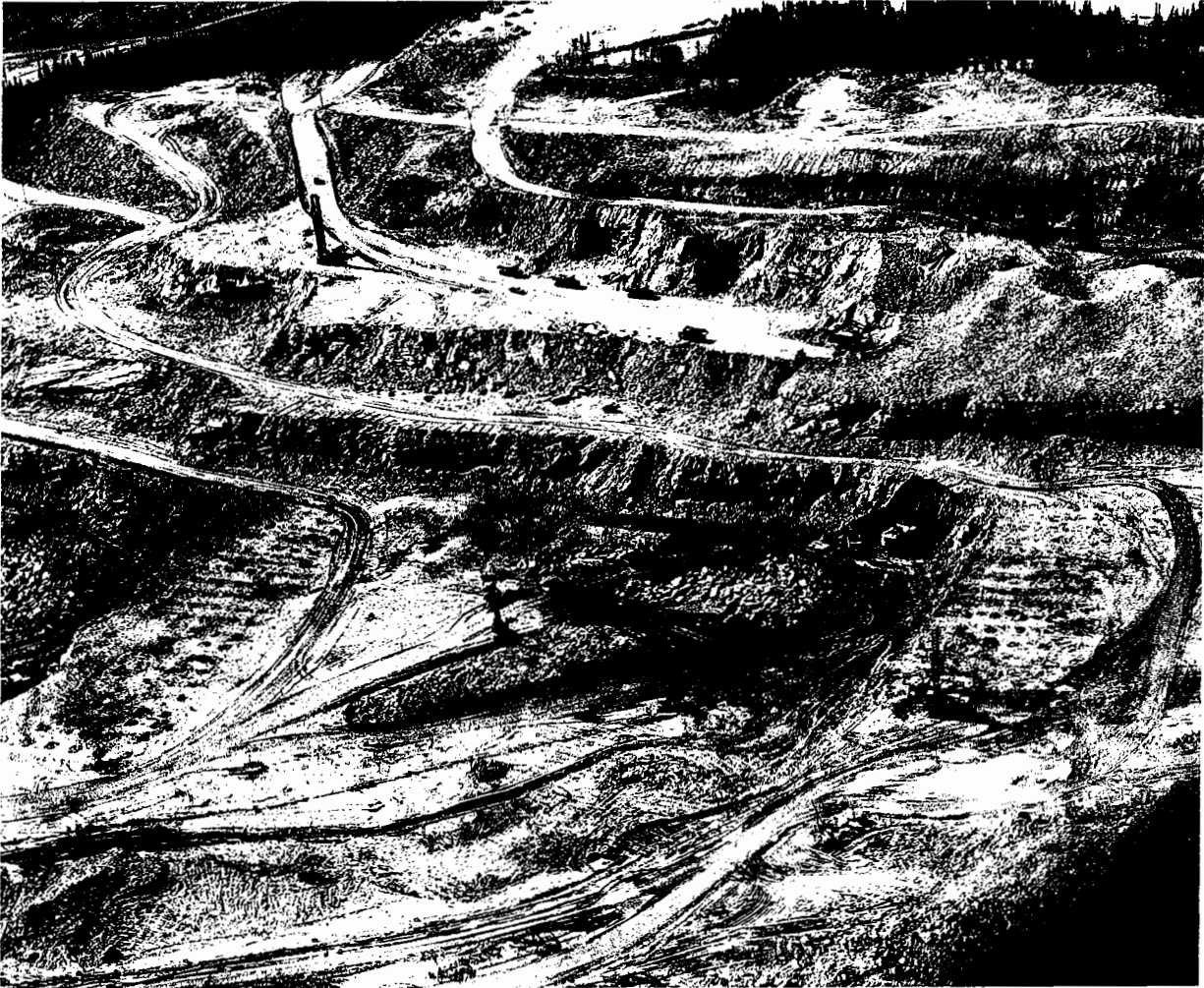
Open pit showing several operations on the many benches. Quebec Cartier Mining Co., Gagnon.
