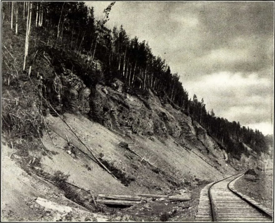
Edmonton sandstone. Cliffs on Canadian Northern railway between Rocky Mountain House and Nordegg, Alberta.
