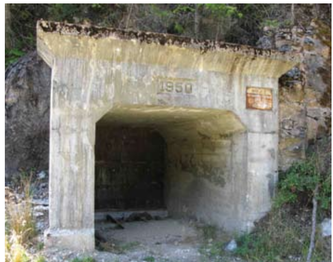
Figure 33. A relict mine tunnel portal at the Bluebell mine on the trail to Galena Bay. Marble cliffs surround the portal. This portal is sealed for safety reasons.
