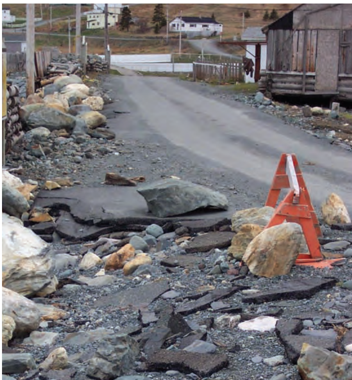
FIGURE 27: Storm-surge damage to road, April 2004, Ferryland, NL.
