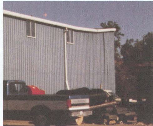
Damage to buildings can be caused by uplift of piles due to frost-jacking.
