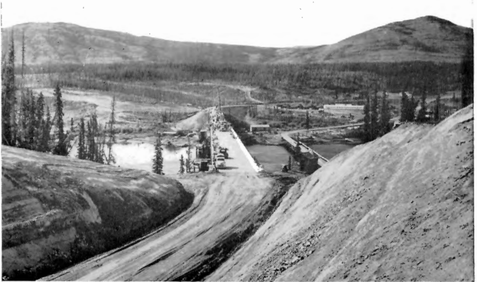
Alaska Highway at Johnsons Crossing, Teslin River, Yukon. Photo by United States Army.
