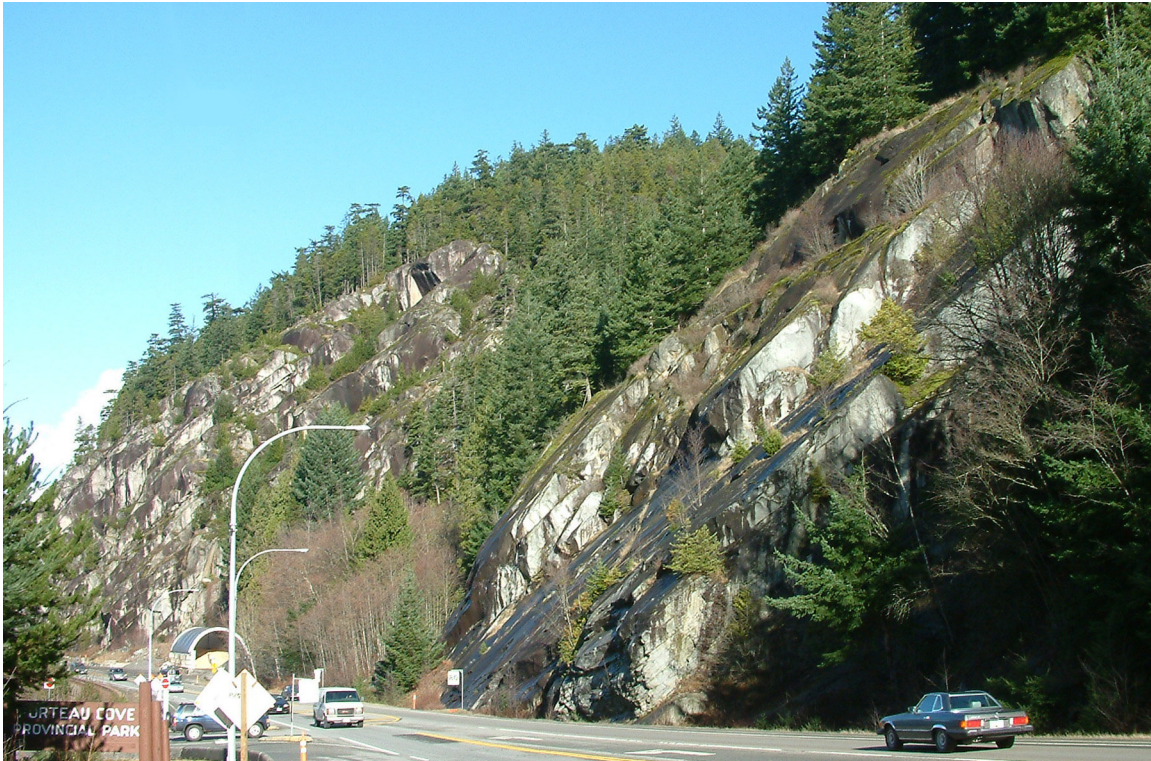
Figure 11. View to the north along Sea-to-Sky highway at Porteau Cove entrance showing the fractures in the quartz diorite dipping toward the road way. These fractures provide sliding surfaces and require engineering works to stabilize the rock.
