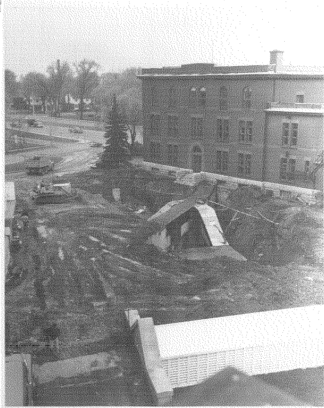
Construction of the new Ottawa vaults. The tunnel connecting the Seismology building to the main Observatory building, the staircases to the two vaults, and the vaults themselves are seen as the backfilling commences.
