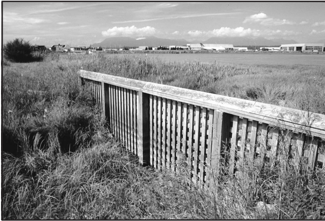
Figure 7. Debris screen at channel opening of constructed marsh, Middle Arm, downstream of No. 2 Road Bridge. Photo by M. Adams. GSC 2003-499
