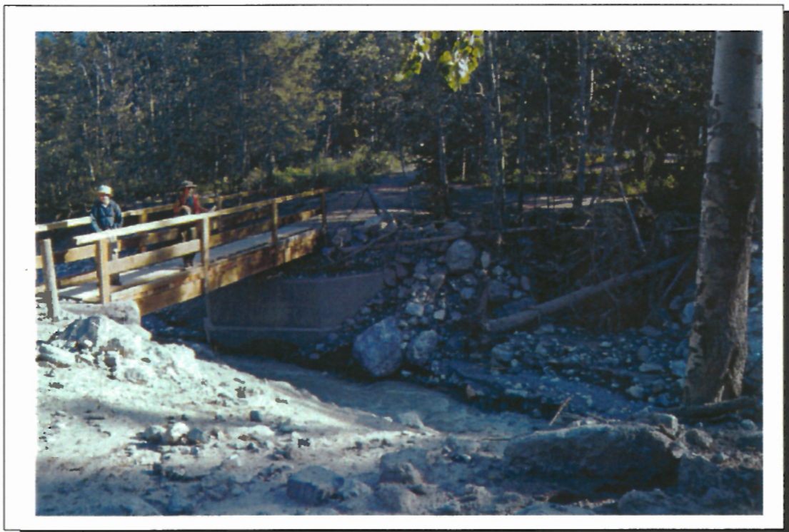
Figure 4.14 The photograph shows a temporary wooden bridge installed over the Five-Mile Creek for hikers. The debris flow undermined the creek bed and completely destroyed the former bridge. Debris flow deposits can be seen on background and foreground.
