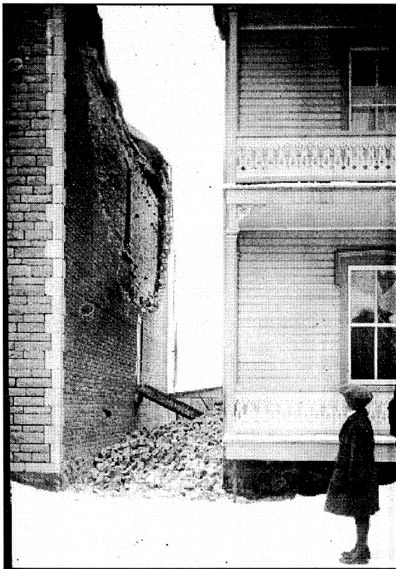
Figure 6. Damaged wall at Shawinigan (Hodgson, 1950).
